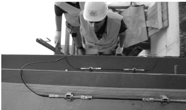
Figure 3: Installation team posing next to two SC-01 already installed and secured in place.
